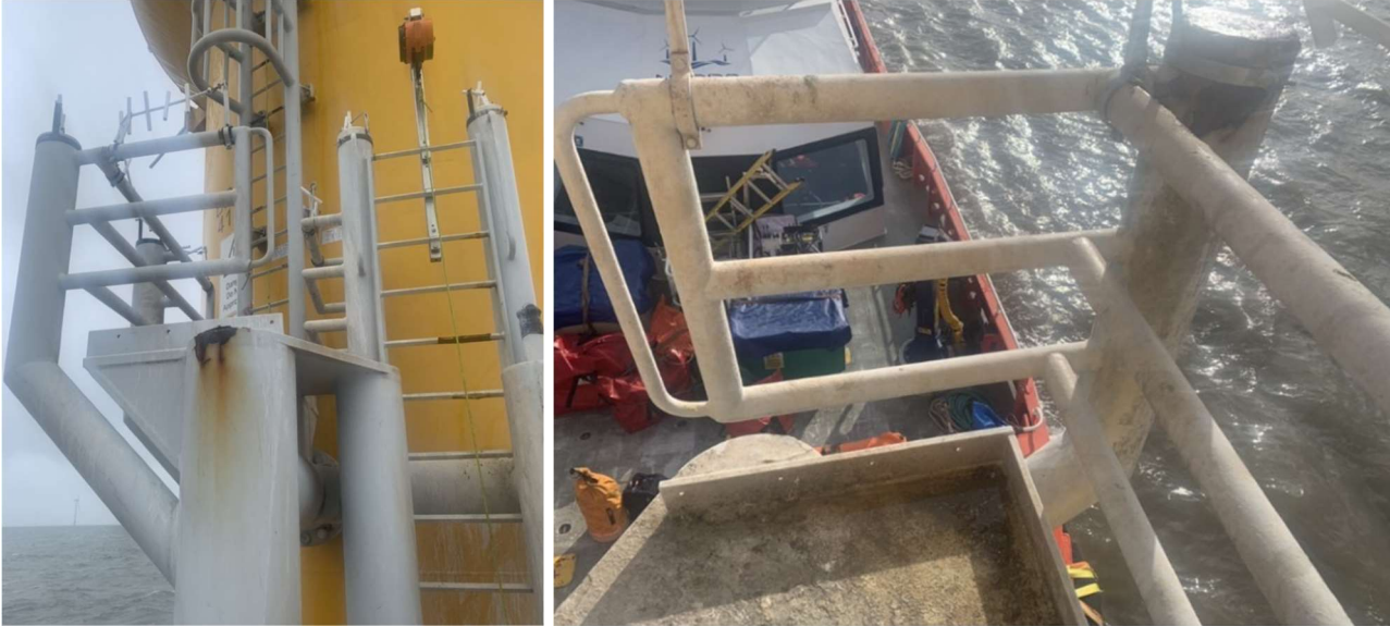
Figure 11: Photos of corrosion at Burbo Bank offshore wind farm (kindly provided by James Almond, Ørsted).
