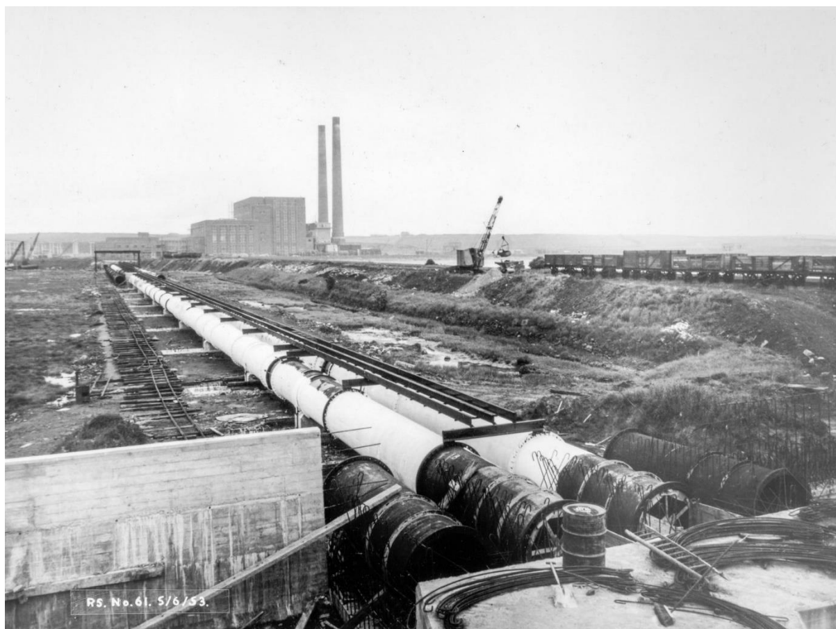
Figure 17: installation of the cooling pipeline for now demolished Roosecote Power Station. Credit: Graham Pinder.
